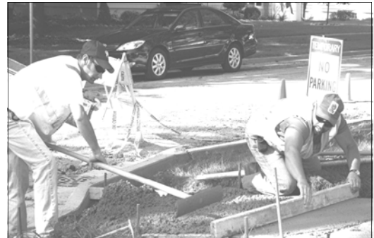
Dept. of Public Works crewmen replace sidewalk at the corner of S. Jackson and Marshall Streets.
