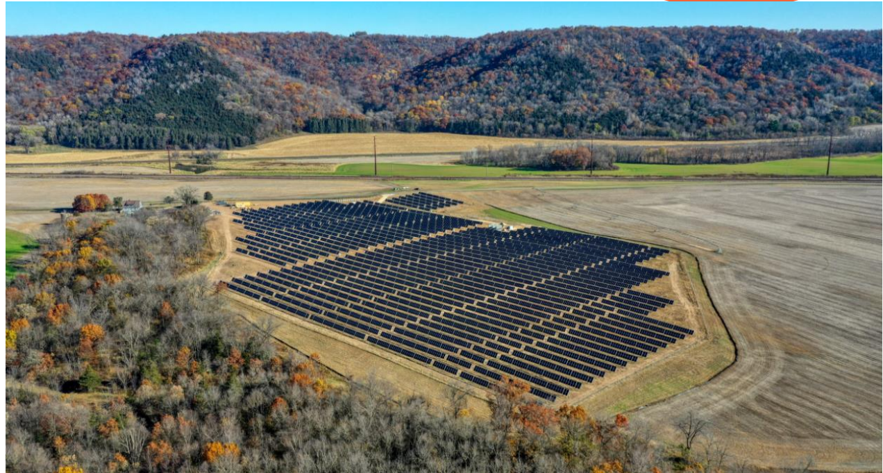
3MW Stromland Solar Project, Cochrane, WI
